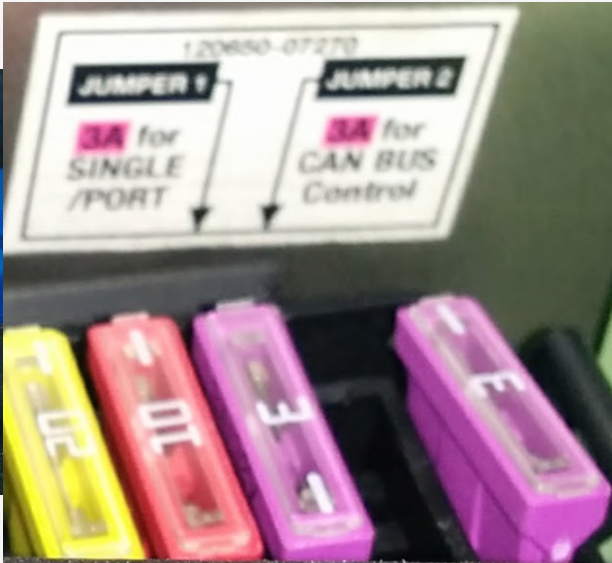
Jumper Fuse for Port & Starboard engines (Single engine labelled (P) Port)
