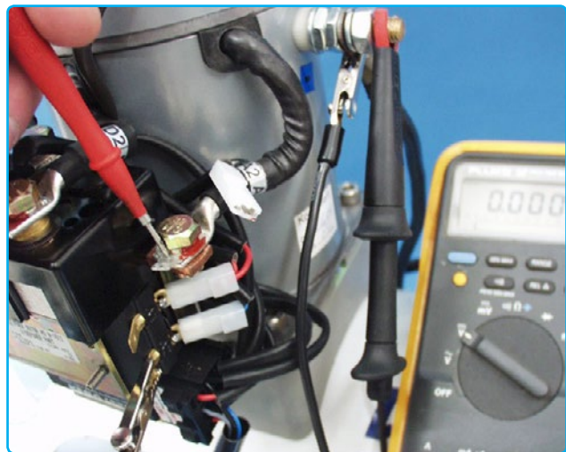
Checking voltage on A2 with ground to blue jumper attached and IPC wire disconnected.
